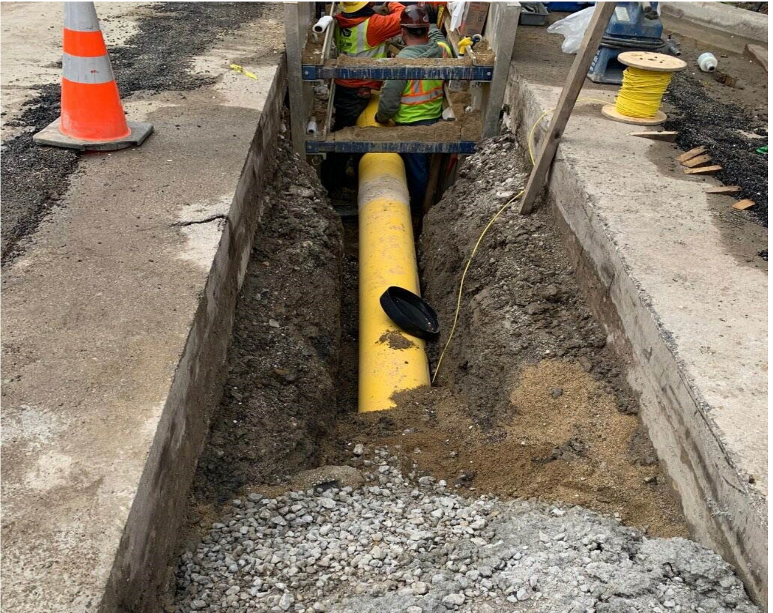
Main installation in Albany Park
